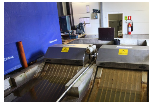
Filtration system at Smolt Farm
